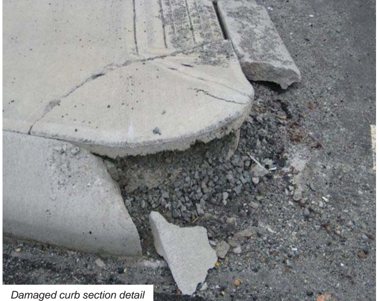
Damaged curb section detail
